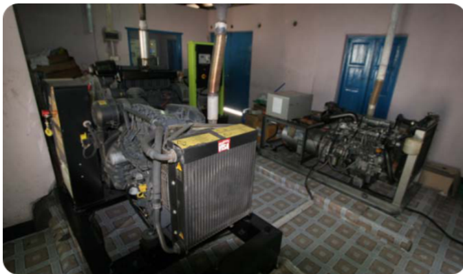
Fig.6- Existing Diesel Generators.
