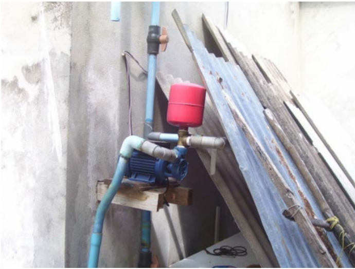
Fig.9-Typical installation of a pressure pump.
